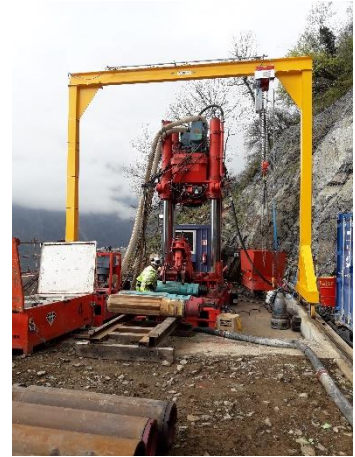
Fig 8. Installation de surface
